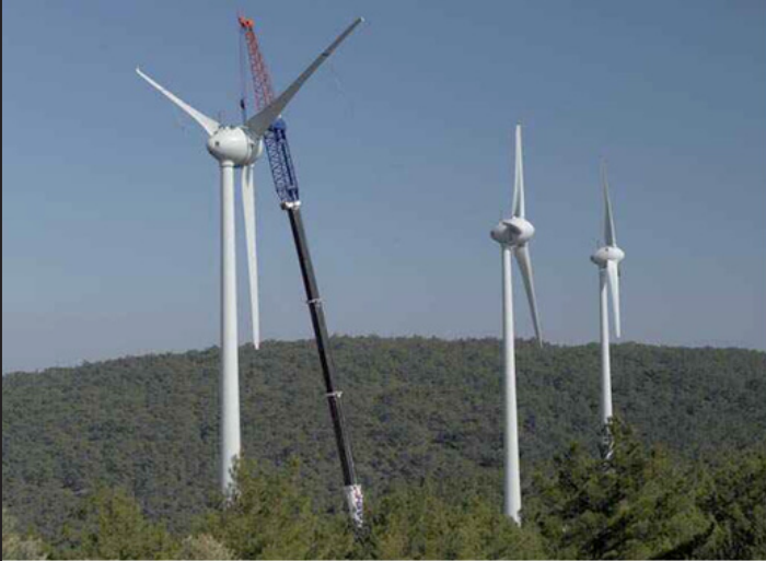
A crane lifting the generator into position for a wind turbine of the same type PASH Global plan to erect on Deadwood Plain
